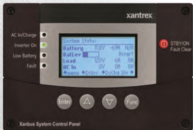
System Control Panel 091-269-008
